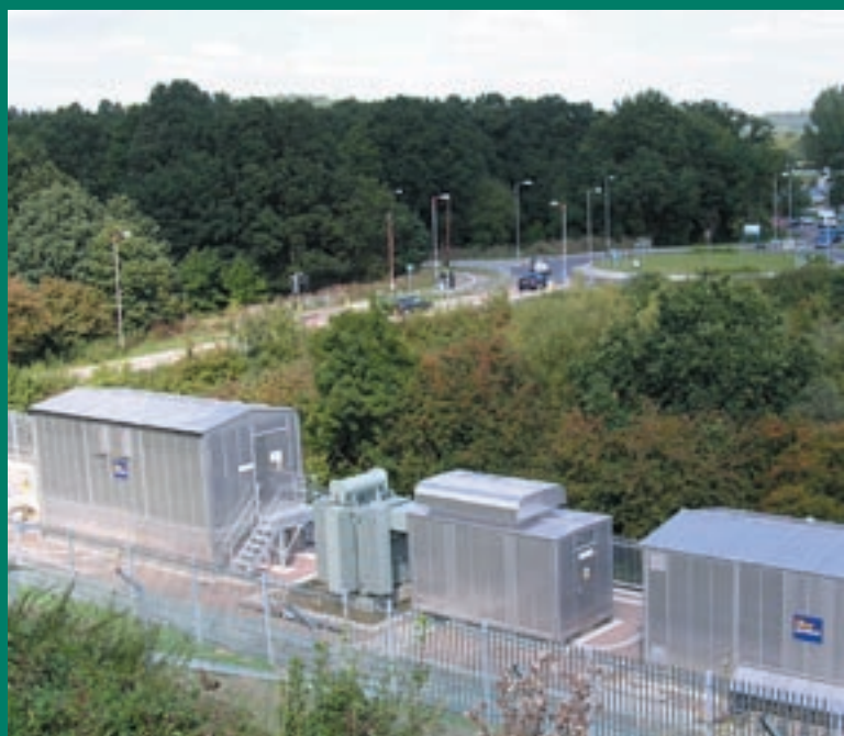
Southern comfort: a completed Power Supply Upgrade substation near Redhill in Surrey
