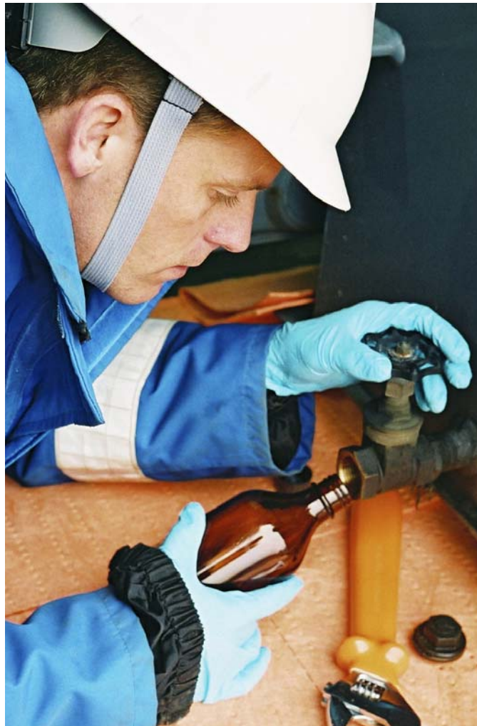
Safety first: an IUS electrical fitter takes a transformer oil sample for condition monitoring analysis
